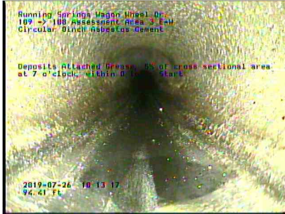
Assessment Area 3 E-W_8302cb01-a044-4ca2-ae67-818e91701811_20190726_101555_039.jpg, 00:08:19, 94.41ft Deposits Attached Grease, 5% of cross sectional area at 7 o'clock, within 8 inch, Start
