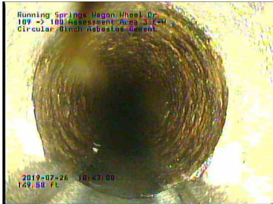
Assessment Area 3 E-W_4e96bbdd-8b01-49ce-9e08-c9614622affa_20190726_104545_804.jpg, 00:18:58, 149.58ft Deposits Attached Encrustation, 5% of cross sectional area from 8 o'clock to 4 o'clock, within 8 inch, Finish
