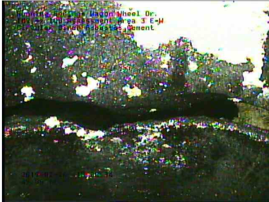
Assessment Area 3 E-W_78f5e56b-d5bf-45eb-8181-22ecf7b8955a_20190726_10111_469.jpg, 00:04:13, 49.46ft Hole Void Visible at 12 o'clock, within 8 inch
