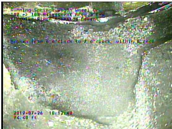
Assessment Area 3 E-W_08ac1a8e-5da5-4675-b115-572704d69e53_20190726_101518_160.jpg, 00:08:08, 94.41ft Broken from 6 o'clock to 7 o'clock, within 8 inch
