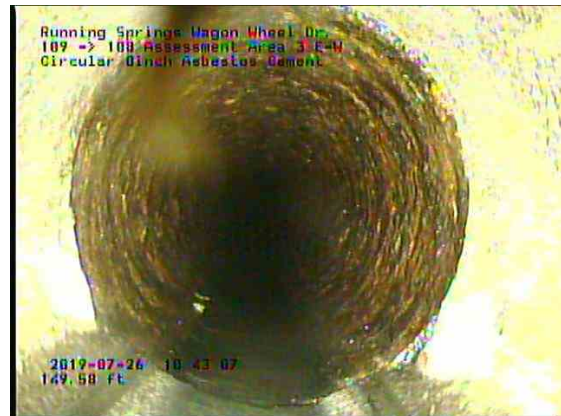
Assessment Area 3 E-W_f5d61b6a-0d56-4274-8eb9-3380554fafcb_20190726_104544_787.jpg, 00:18:56, 149.58ft Deposits Attached Grease, 5% of cross sectional area at 5 o'clock, within 8 inch, Finish
