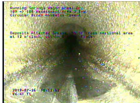
Assessment Area 3 E-W_d6e33a41-d3fc-49f3-a18b-8aead2840e17_20190726_101529_811.jpg, 00:08:16, 94.41ft Deposits Attached Grease, 5% of cross sectional area at 12 o'clock, within 8 inch, Finish
