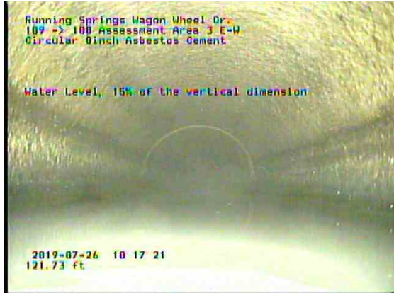
Assessment Area 3 E-W_a07849ee-8ffa-4858-bad8-1dfc7f52cb50_20190726_101958_689.jpg, 00:11:08, 121.73ft Water Level, 15% of the vertical dimension
