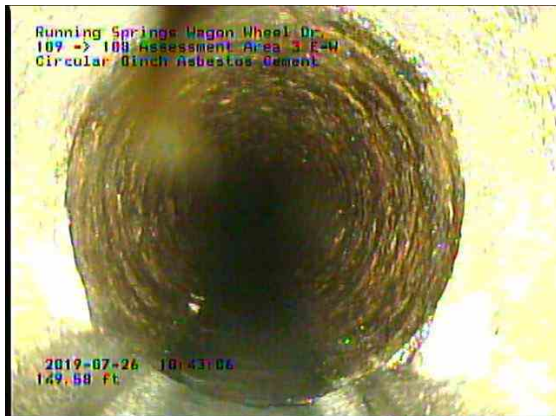
Assessment Area 3 E-W_2d459580-2ad1-4005-8d33-e545637c9d9c_20190726_104543_860.jpg, 00:18:55, 149.58ft Deposits Attached Grease, 5% of cross sectional area at 7 o'clock, within 8 inch, Finish
