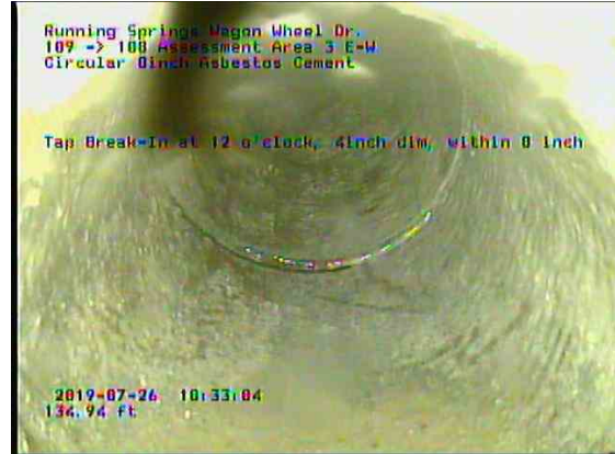
Assessment Area 3 E-W_ceda1ad6-48f9-471e-92e7-7d4e8ecfc9a2_20190726_103541_995.jpg, 00:13:29, 134.94ft Tap Break-In at 12 o'clock, 4inch dim, within 8 inch
