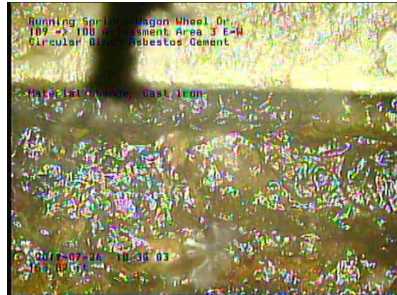
Assessment Area 3 E-W_27eceda3-1b13-4d5c-9af1-7c387b50a2e6_20190726_103740_601.jpg, 00:15:03, 153.02ft Material Change, Cast iron / 8"
