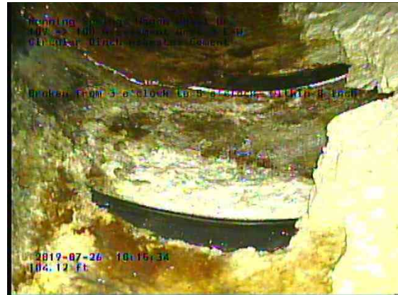
Assessment Area 3 E-W_a98b0ae1-aa09-403e-8978-00b09f5d5bc6_20190726_101811_257.jpg, 00:09:31, 104.12ft Broken from 3 o'clock to 5 o'clock, within 8 inch
