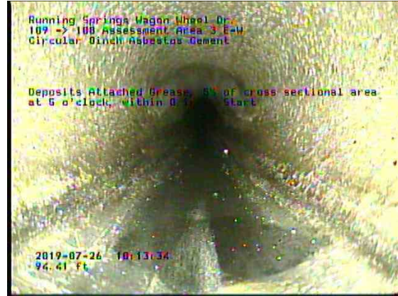
Assessment Area 3 E-W_f1924e49-2210-4ff9-bcae-de53c4ee99c8_20190726_101611_984.jpg, 00:08:22, 94.41ft Deposits Attached Grease, 5% of cross sectional area at 5 o'clock, within 8 inch, Start
