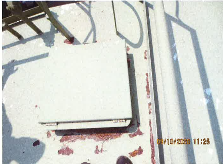
Roof of Luring Pines tank (external) Coating is peeling
